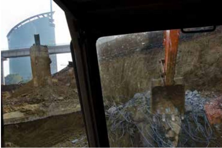
Work in progress at an IL&FS construction site for DLF underpass. The Gateway tower can be seen in the background.
